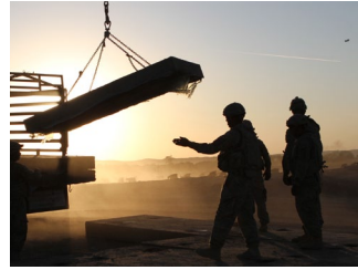
Soldiers worked from dawn to dusk on the construction of Lukenbach Crossing.
