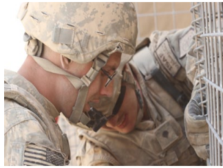
PFC Robert Green and SPC Christopher Mohney assemble last section of HLZ wall.
