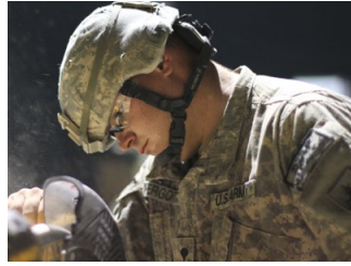
SPC Lander Hergott with 623rd EN CO cuts lumber for a new building project.
