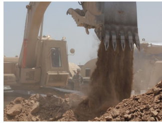
Bucket loader operated by SGT Fowler prepares a pit for waste tank installment.
